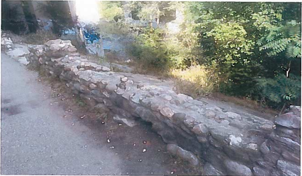
Franklin Mill Riveredge Trail Stone Wall – missing wall section and missing wood timber top rail
