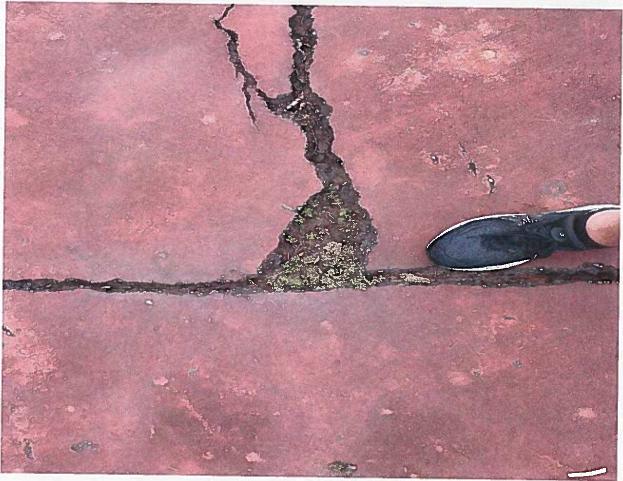
Al Lease Park Basketball Court Cracking
